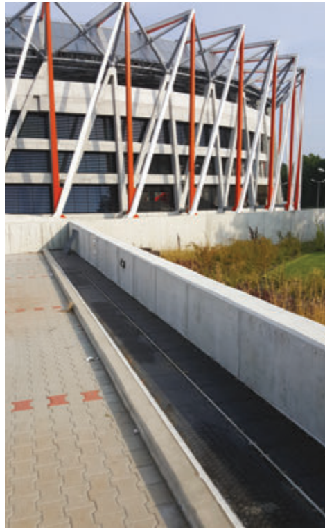
City Stadium Białystok AS-300 drainage channels with cast iron covers
