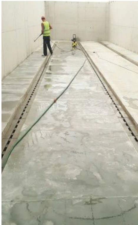
Waste Treatment Plant
